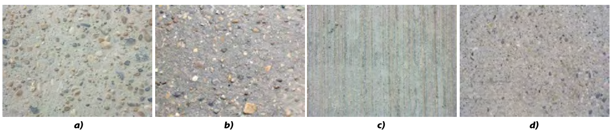
Fig.6. Pictures of the water jet scrubbed concrete (a. initial state, b. after two years); pictures of the broomed surface (c. initial state, d. after 2 years)
