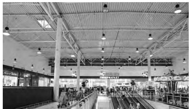
Fig. 6. The illumination system before reconstruction – permanent artificial light IDs. Light sources are HP MHLs
