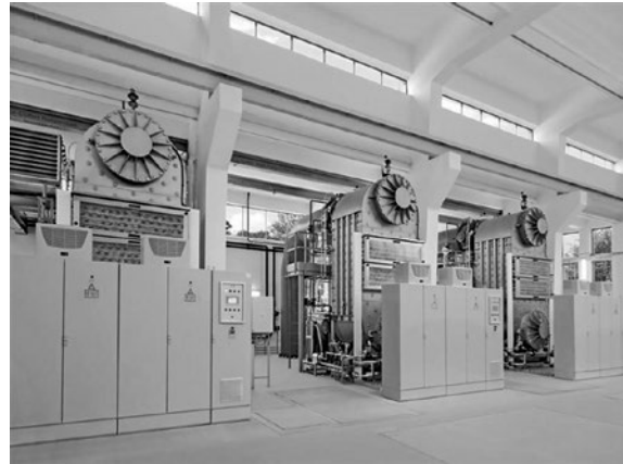
Fig. 2. UV disinfection station of surface water (Budapest, Hungary); number of lamps type ДБ 350 is 600, total power consumption is 210 kW
