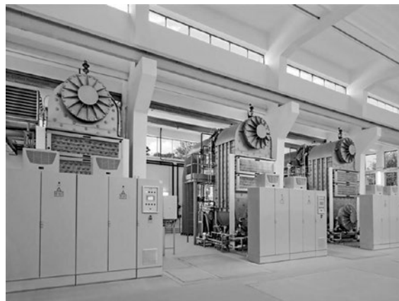
Fig. 2. UV disinfection station of surface water (Budapest, Hungary); number of lamps type ДБ 350 is 600, total power consumption is 210 kW
