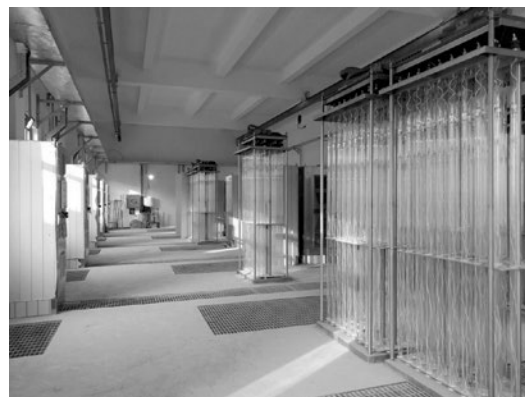
Fig. 4. UV disinfection station of waste water (Beijing); number of lamps type ДБ900HO is 864, total power consumption is 700 kW
