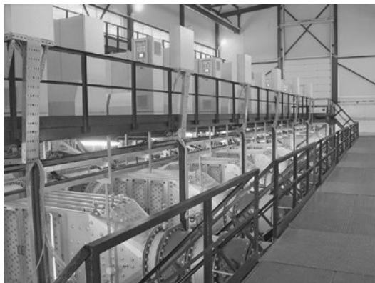
Fig. 1. UV disinfection system of the Northern waterwork (St. Petersburg) of 1,584,000 m 3 /day productivity (number of lamps type ДБ 350 is 3888 with total power consumption equal to 1.36 MW)
