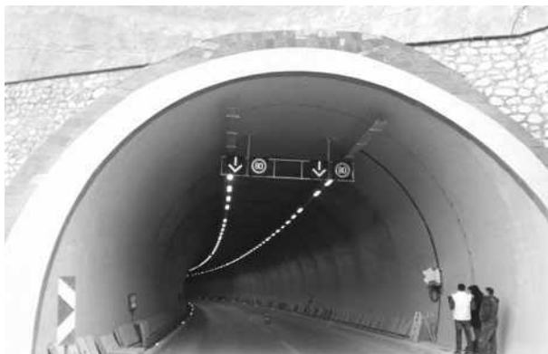
Fig. 5. Illumination of the Buzlupınar tunnel using LED luminaires
