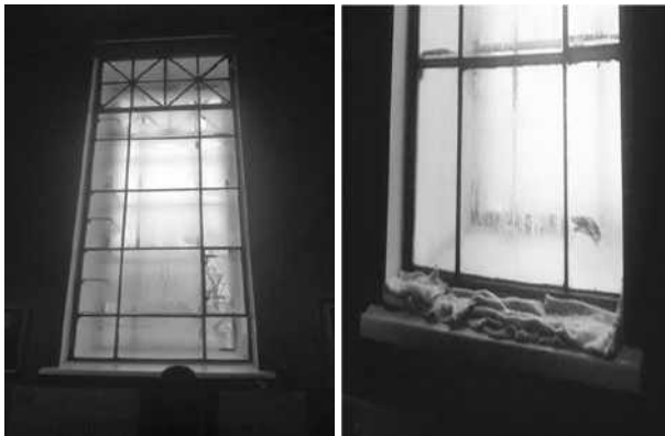
Fig. 3. Condensate formation on the inner surface of translucent cladding
