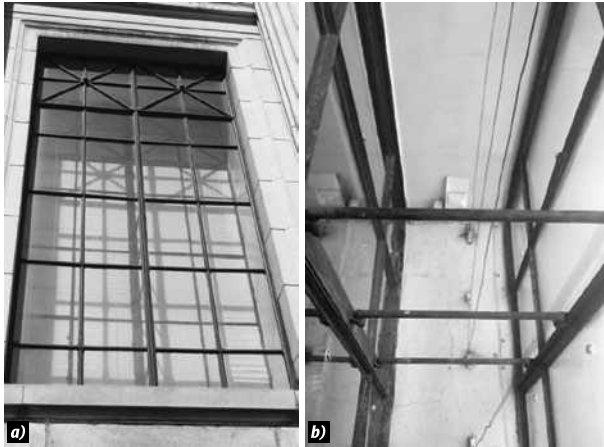
Fig. 2. Historical windows in the major building of the Pushkin State Museum of Fine Arts: a – view from the outside, b – metal bonding (“ladder”) between external and internal sashes
