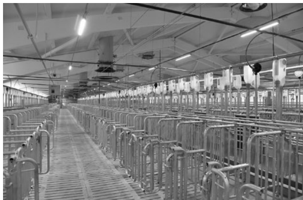
Fig. 3. LED lighting in pig-breeding complex [7]
