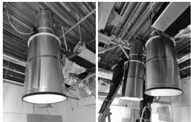
Fig.7. HLC “Solar LED-S” in the “Meeting room “ (installation process). ALB is located in the space of the technical floor, located above the ceiling of the “Meeting room” under the roof (internal design)
